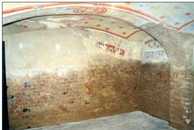
Povodeň 2002. Poškozená modlitebna z doby ghetta. Flood in 2002. Damaged prayer room from the time of the Ghetto.
